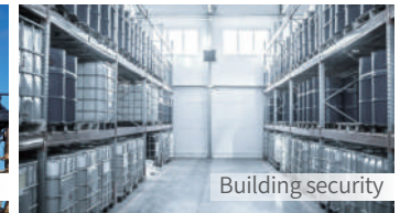
Electrical equipment inspection
