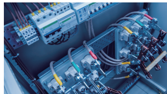
Electrical equipment monitoring
